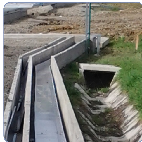
Linee interrate in complesso industriale - Firenze (FI) Underground lines in industrial complex - Florence (FI)
