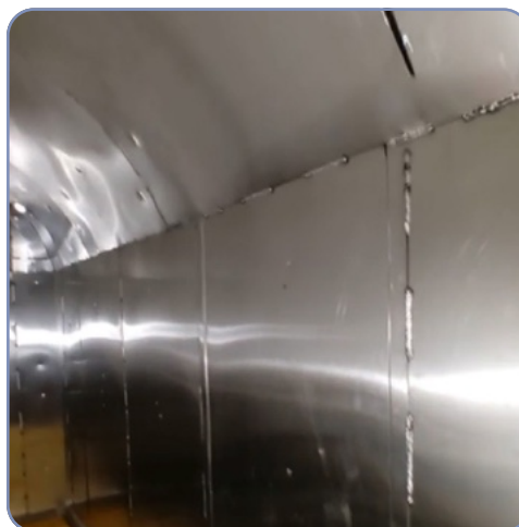
Cabina ente distributore - Roma (RM) Distributor cabin - Rome (RM)
